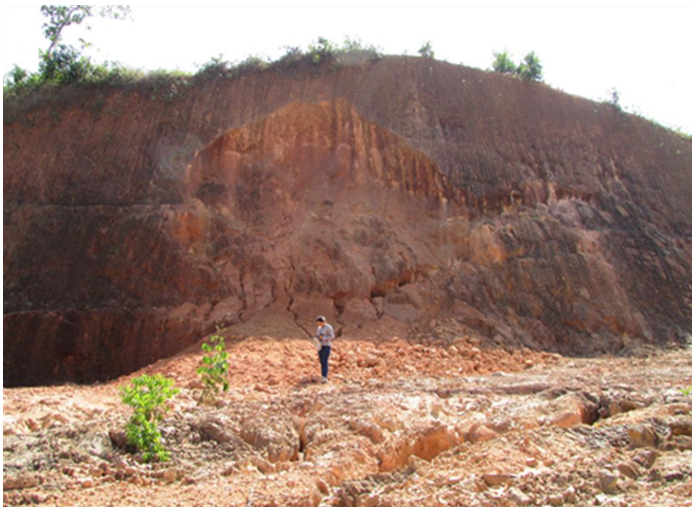
Photo – 4: Extensive Slope Cut near Indamogru Village (Toposheet No 48P/05). The material has already started moving due to rain.
