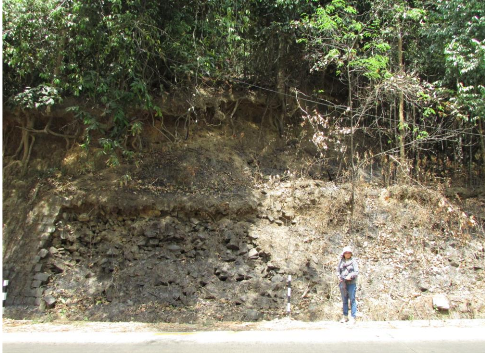
Photo – 15: View of debris slide along NH – 75 (formally known as NH – 48) in the east of Shradigadi (Slide Name – KAR/HAS/48P09/2016/11) (Toposheet No – 48P/09). The retaining wall has started to collapse due to movement that clearly suggests that the slide is active.
