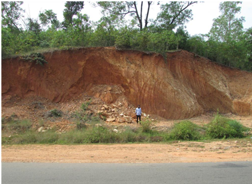
Photo – 3: Extensive Slope Cut along NH – 75 (formally known as NH – 48) in the east of Uppinangadi (Toposheet No 48P/05).
